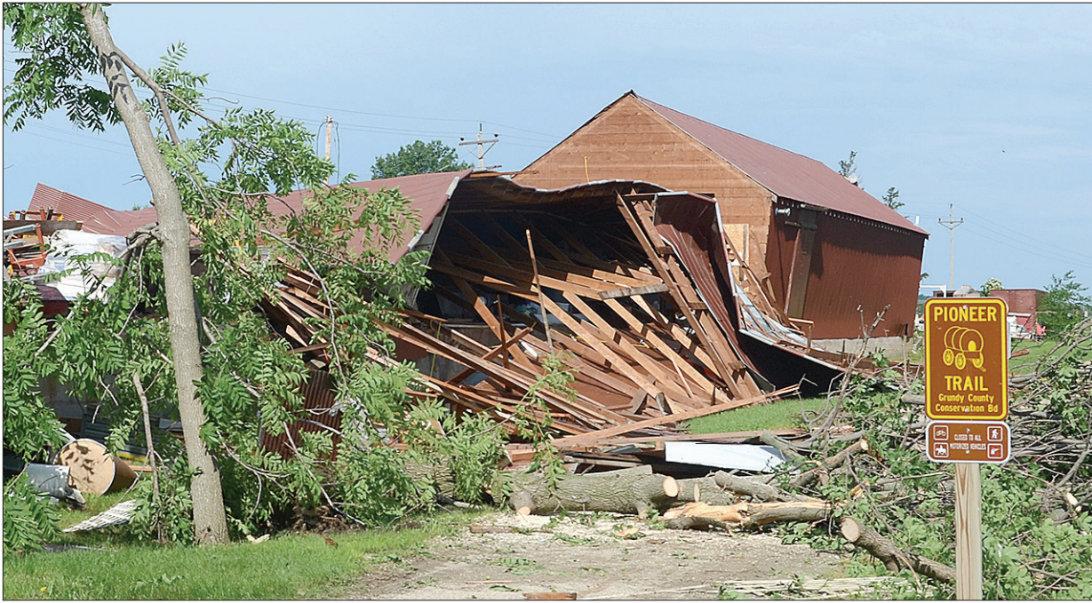
Buildings along the Pioneer Trail in Morrison received significant damage in the June 29 storm. (John Jensen/The Grundy Register photo)
